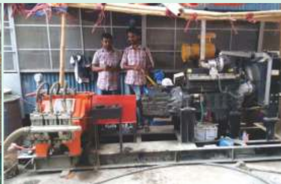
High Pressure Jet Grout Pump System
